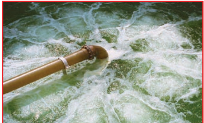
MIXING AND AERATION IN pH CONTROL TANK
