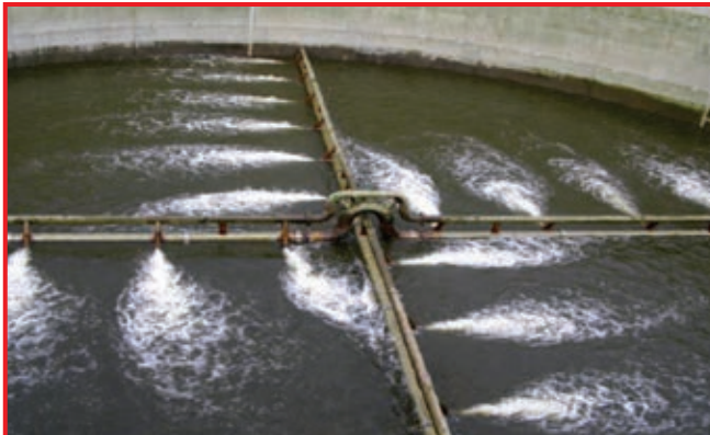
JET MIXING IN EQUALIZATION TANKS
