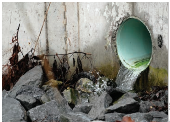
Water resource recovery facility discharge outfall
