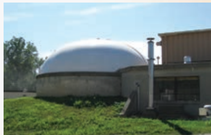
Digester Gas Holding Cover
